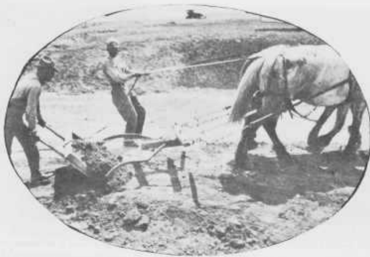
Two men were needed to operate a fresno. With this operation 1,000 yards of dirt were moved daily.
