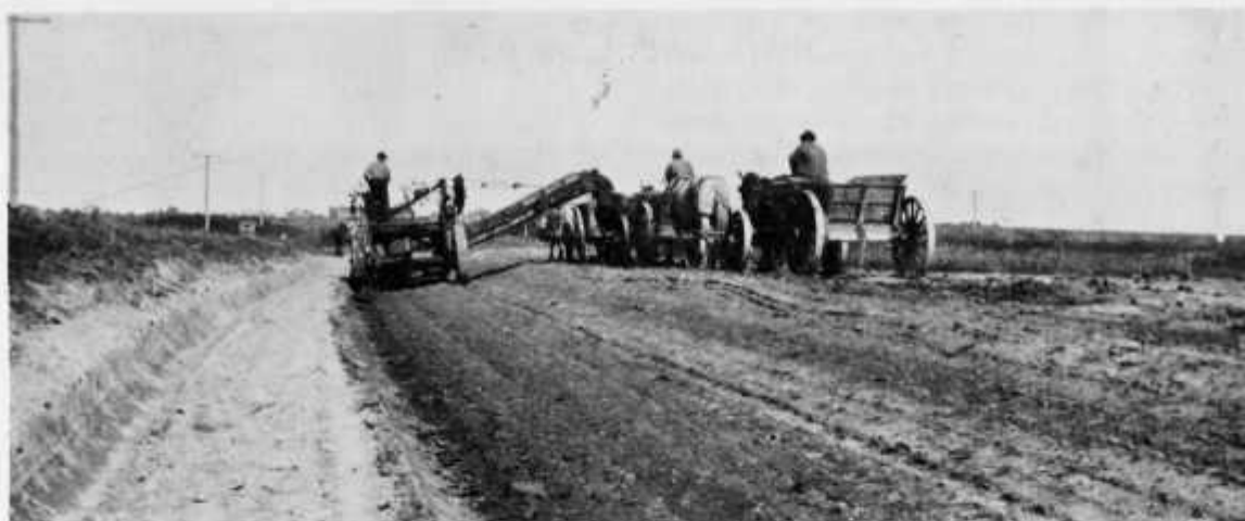
Pictured is some of the Campbell Construction Company workers at St. John, North Dakota in 1928. Atop the "cat" is Maynard Brown.
