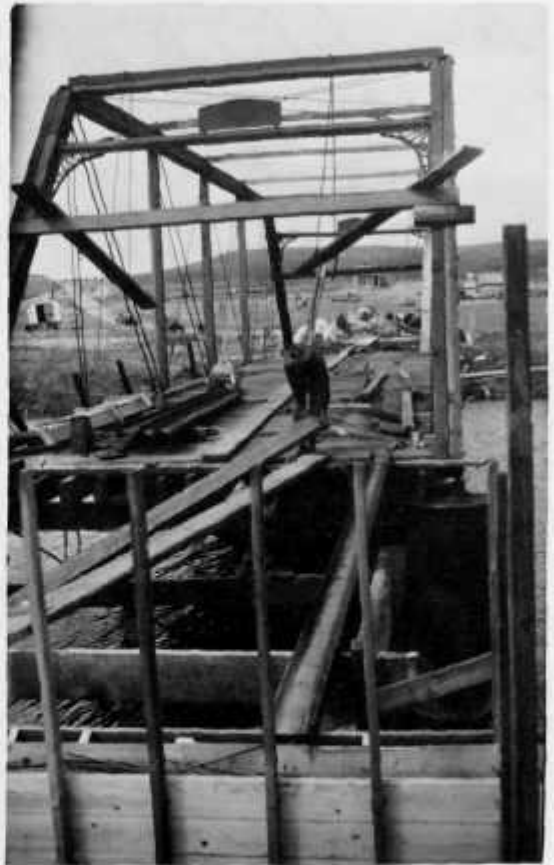
Building of the "Red" bridge across the Sheyenne River in Freeborn Township, 1907.
