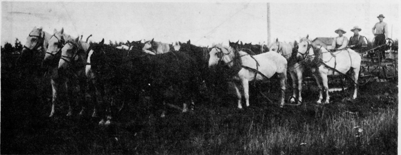
This is the way roads were built in the early days. This is looking North 17 miles west of Bottineau at the corner known as the H.J. Hanson farm. The mile being built is from what is now No. 5 and south one mile to the Herbert Thompson farm. The building and trees in the back ground is the homestead of Lewis Tiegan, this is now all field.
