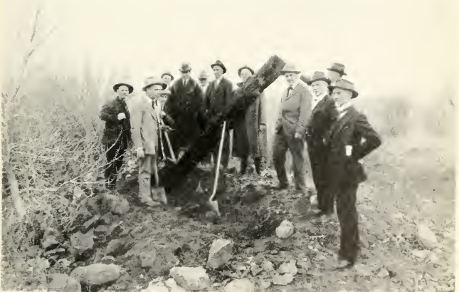
EXCAVATING A LOG (NOVEMBER 9, 1922) THAT FORMED A PORTION OF THE CRIBBING FOR ONE OF THE PIERS OF OLD PLATTE BRIDGE. BUILT IN 1858-9.
